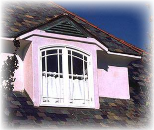
Window shape and mullion pattern are both useful elements for creating character.
